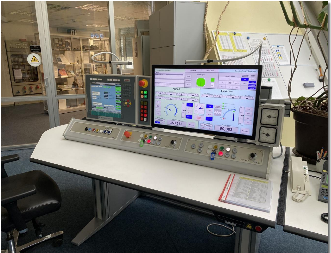
The new touch panel for the main axes control (right), besides the touch panel for the subreflector – in the control room of the telescope (picture by H. Homburg).
