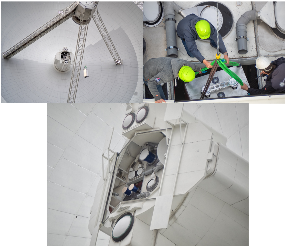
Top: Transport and Installation of the receiver in the secondary focus cabin. Bottom: The new receiver in the telescope (the two blue horns in the center).
